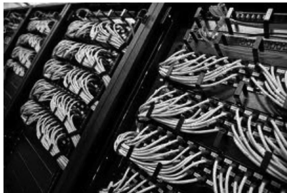
FIGURE 10.2 Networking infrastructure in data centers.
